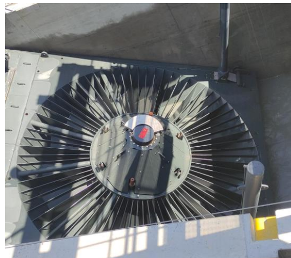
Turbine VLH installée
